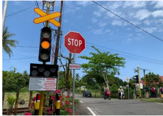
Figure 1. Early warning system installed at a railway level crossing in Indonesia [1].
