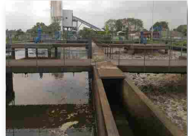
Wastewater treatment facilities
