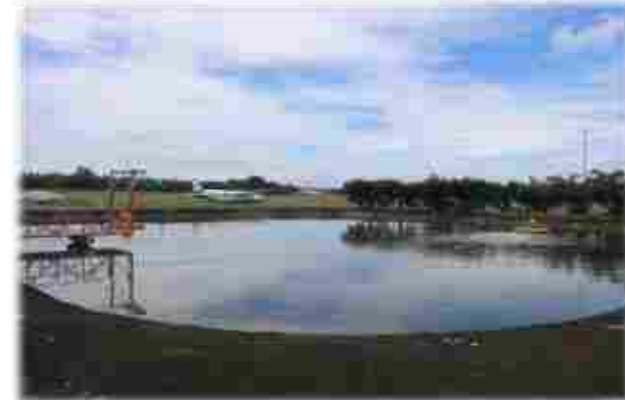
Wastewater treatment facilities
